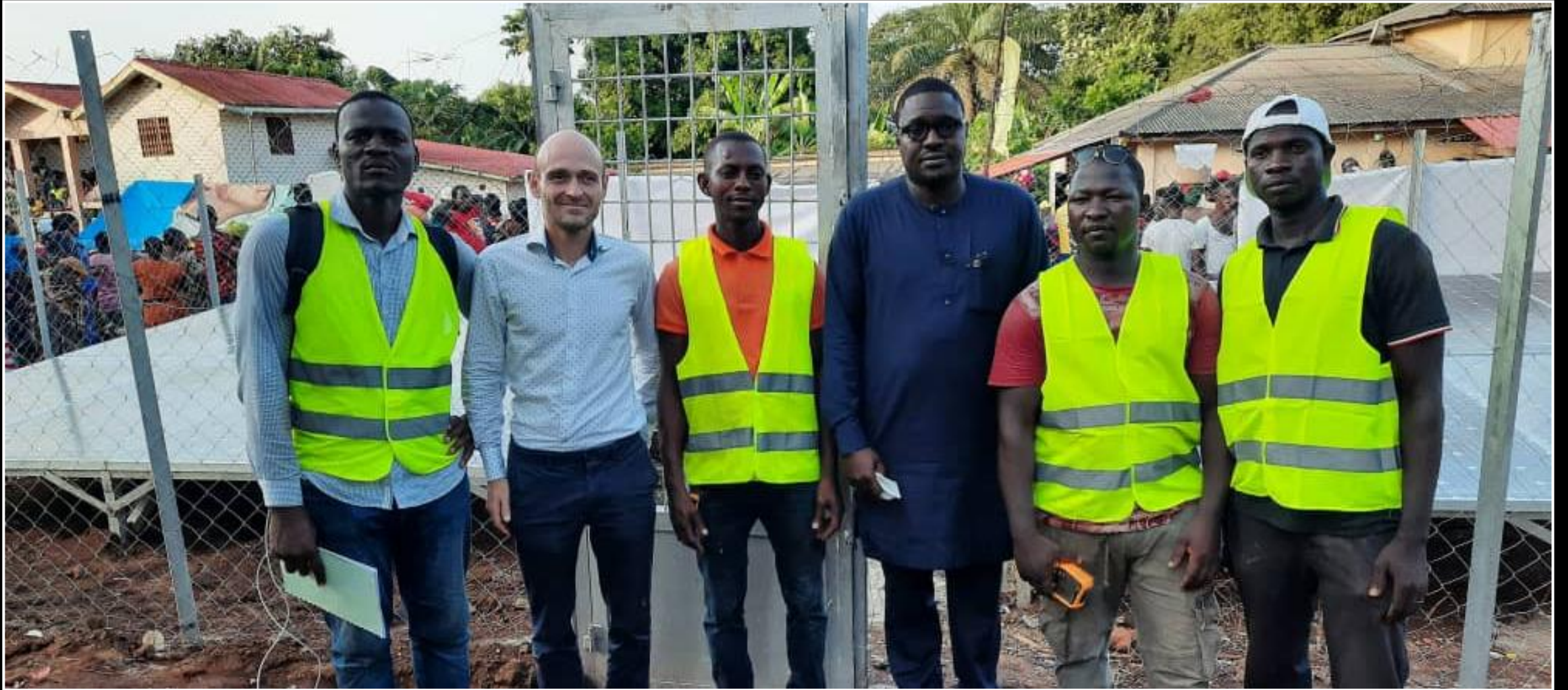
Fencing of PV Module Hub
